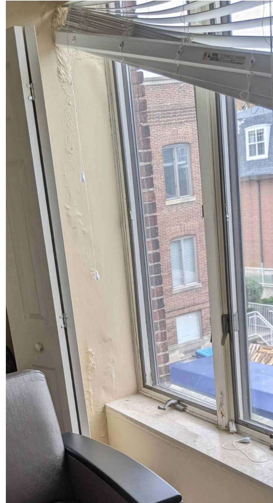
TYPICAL WINDOWS TO BE REPLACED BY WINDOWS A/B/C/J/L. SEE ELEVATIONS AND ELEVATION PHOTOS FOR WINDOW TYPES AND LOCATIONS.
